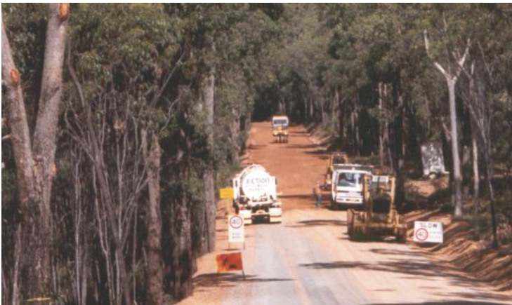
Road construction with Phytophthora Dieback infected soil or gravel can lead to the introduction of the disease into adjacent bushland.
